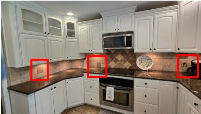
No GFCI at outlets
