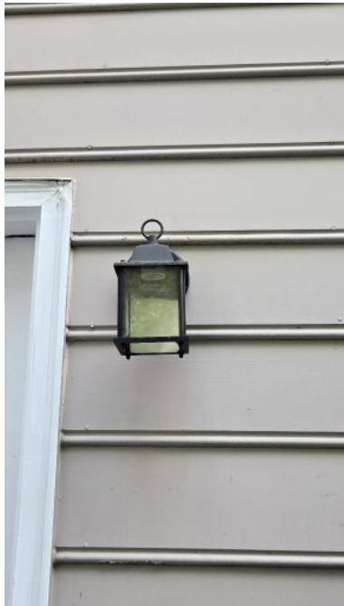
Missing light bulb
