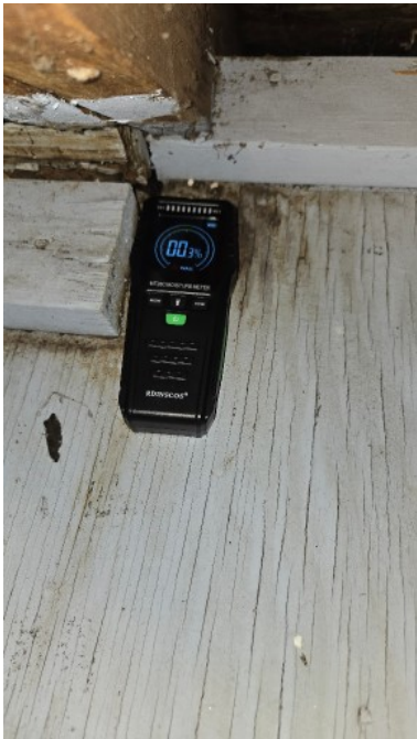
No moisture detected
