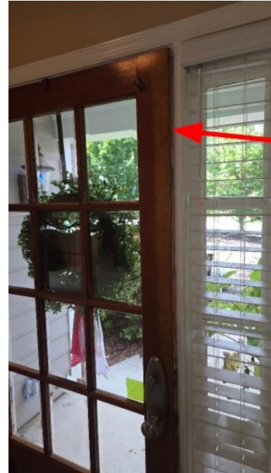
Door sticks to the frame
